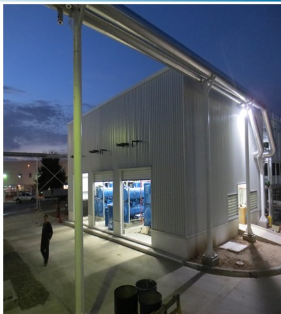
Tecochill chillers keep Mexican factories cool, despite often unreliable grid power.
