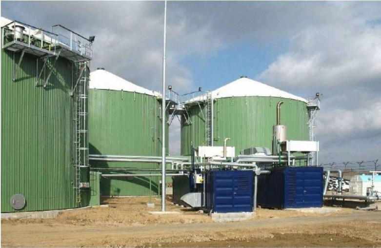
TEDOM Quanto units fueled by renewable biogas provide power and heating services to over 100 sites worldwide.
