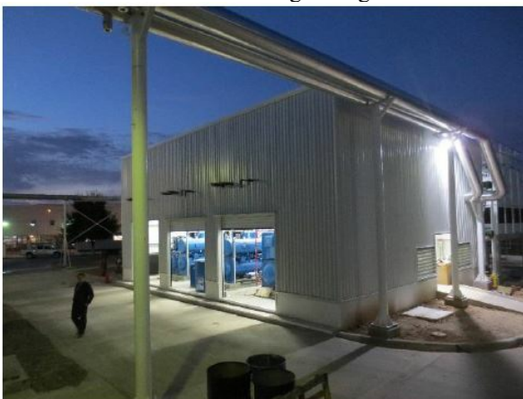
TECOCHILL chillers keep Kohler's Mexican facility cool, despite often unreliable electric service.
