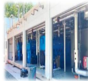
1200 ton Tecochill Modular Chiller Plant (MCP) for cannabis cultivation facility in MA
