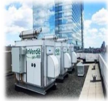
300 kW Microgrid in New Jersey
