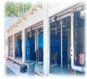
1200 ton Tecochill Modular Chiller Plant (MCP) for cannabis cultivation facility in MA
